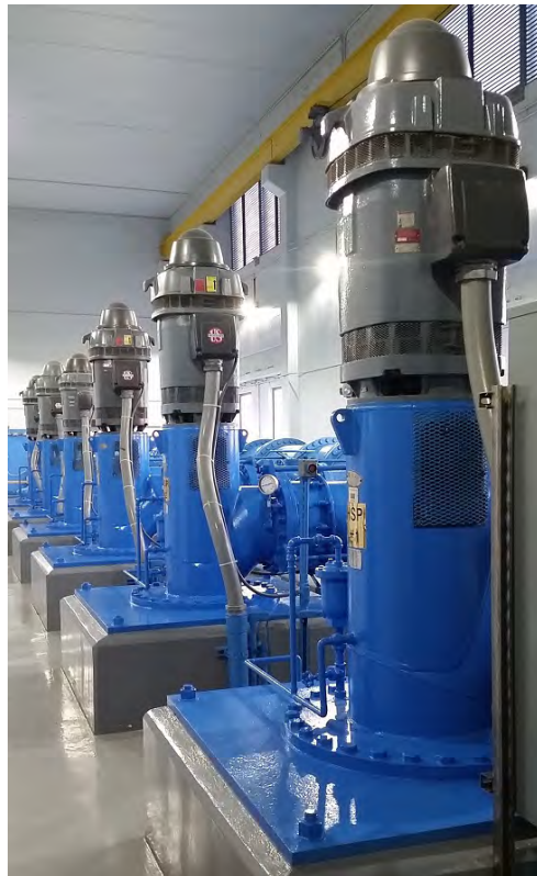
These six high service pumps are used to transport treated water from ground storage tanks into the distribution system to service customers.
