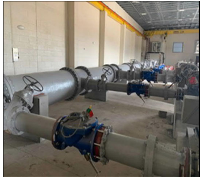
Waterset Reclaimed Water Pump Station and Storage Tank
