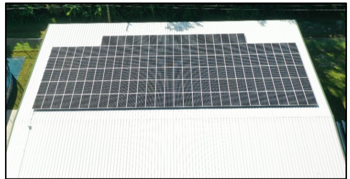
Solar Panels – Ruskin Recreation Center
