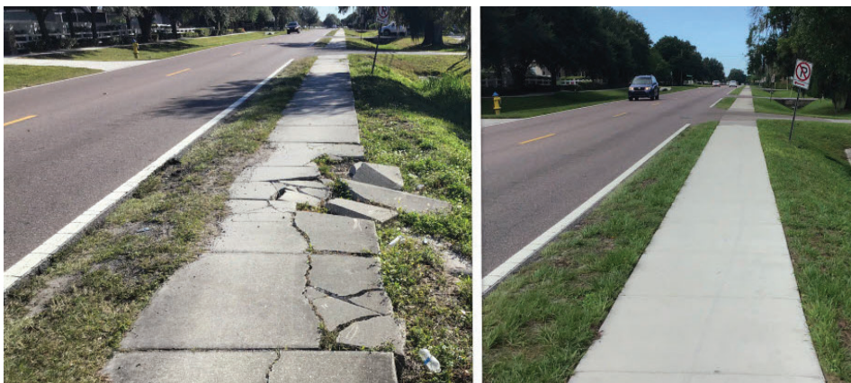
County staff designed and replaced the sidewalk adjacent to the ditch line with reinforcing mat to prevent future erosion issues.
