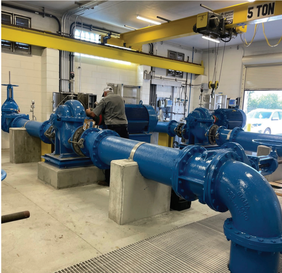
A County employee works on pipes in the South County Pump Station.
