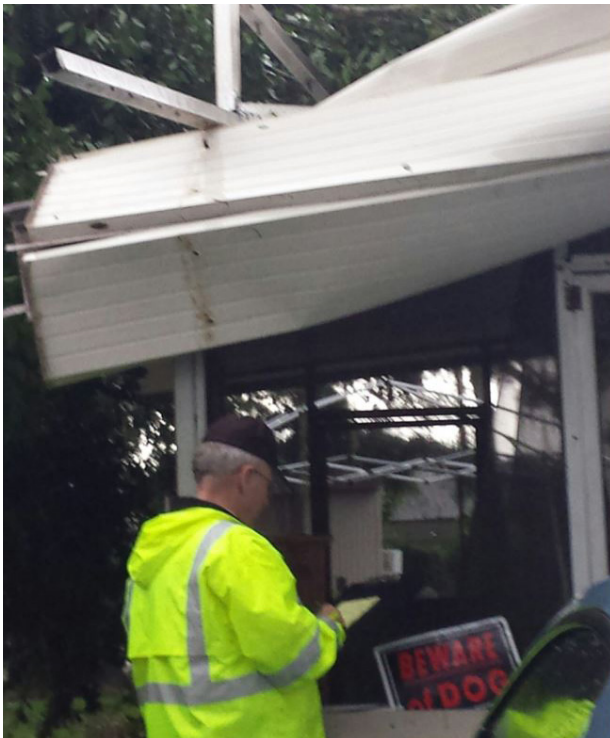
A Code Enforcement officer conducts a damage assessment after a storm.
