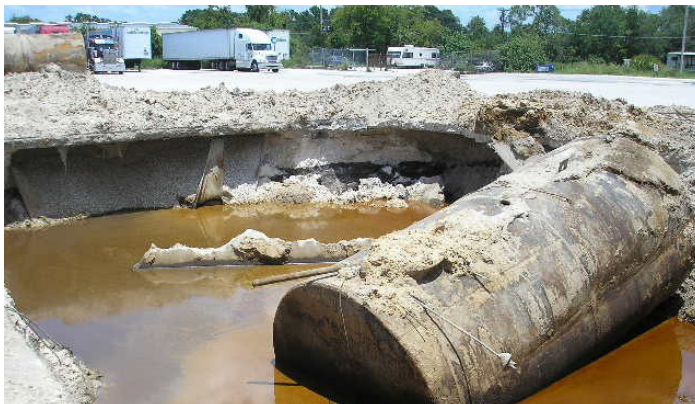
The EPC is helping clean up over 2,000 leaking petroleum tanks threatening ground water.
