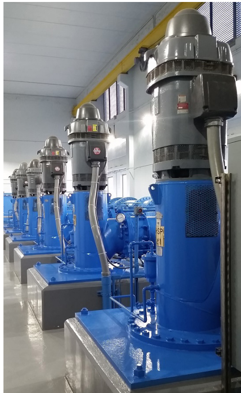
These six high service pumps are used to transport treated water from ground storage tanks into the distribution system to service utility customers.
