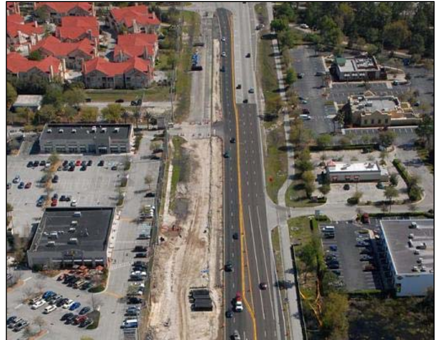
An aerial view of Bruce B. Downs-Palms Springs Blvd to Pebble Creek Dr East of I-75.
