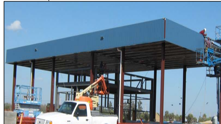
Construction of this entrance canopy is just one of many improvements made to the South County Transfer Station.
