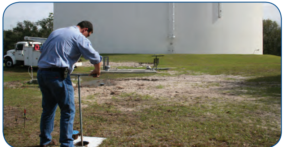
A staff member conducts valve maintenance for the County's drinking water system.
