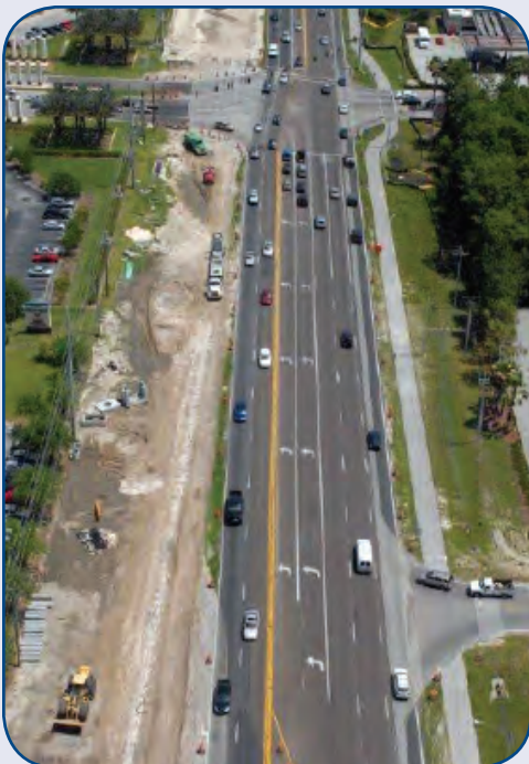
Construction of a new lane on Bruce B. Downs Boulevard between Palm Springs Road and Pebble Creek Road.
