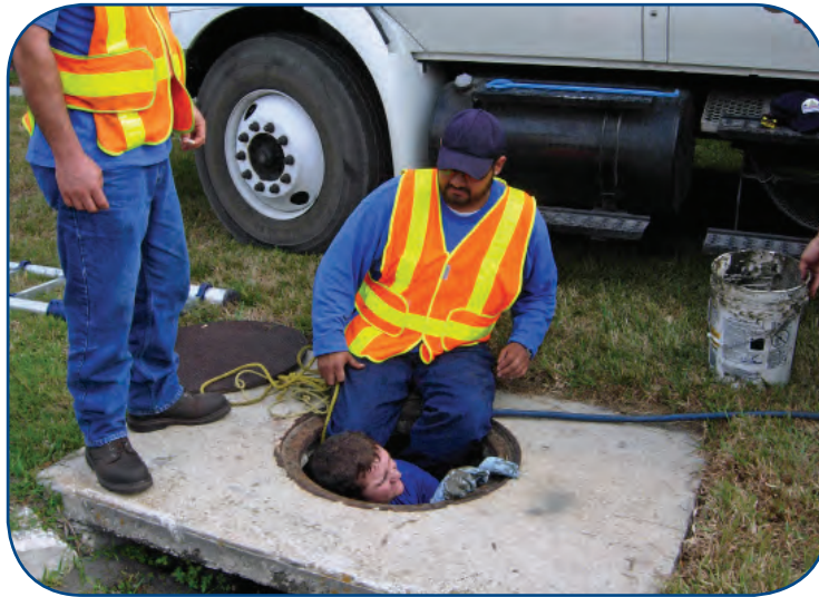
Workers investigate the stormwater pipe system to prepare for maintenance and repairs.
