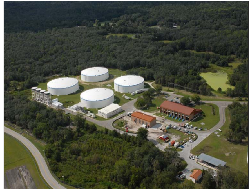
Lithia Water Treatment Plant
