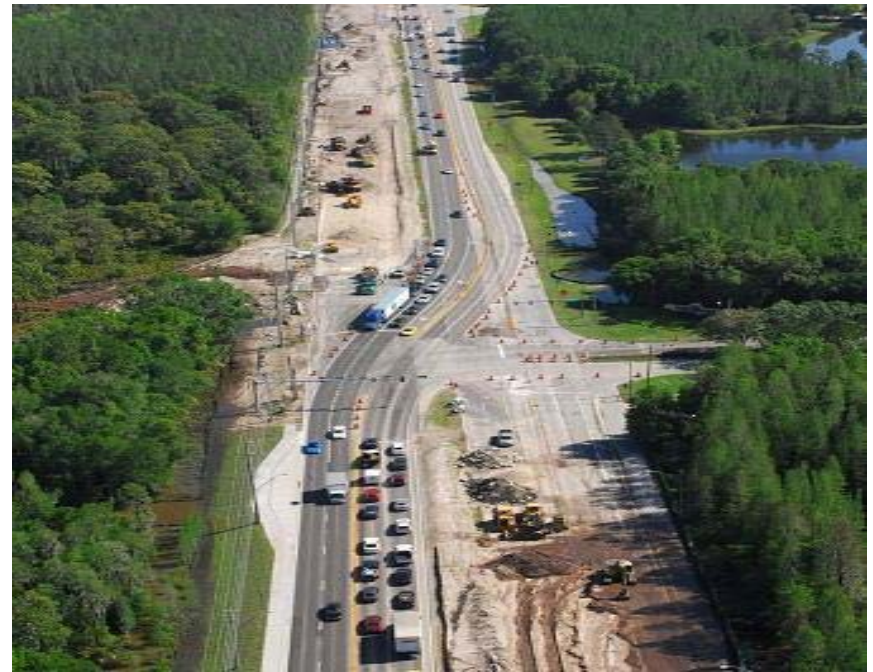
Bruce B. Downs (Palm Springs to Pebble Creek Drive South) Road Widening
