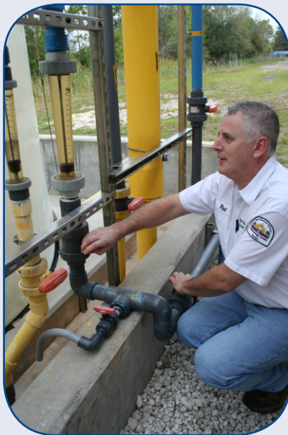
A Public Utilities Department staff member makes water treatment adjustments to ensure clean drinking water.
