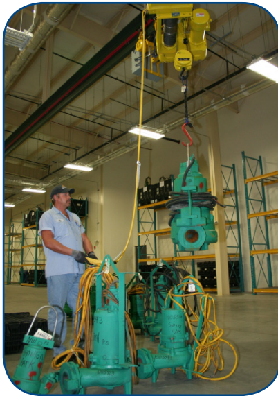
A staff member puts in a hard day's work in the submersible pump maintenance shop.
