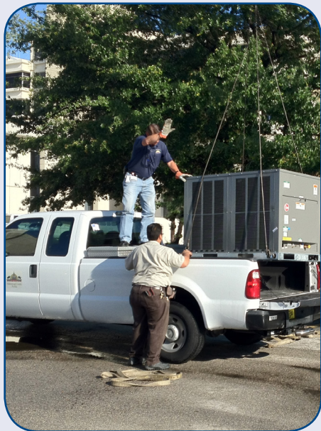
Staff members prepare for a crane to lift a new air conditioning unit for installation on the roof of the administration building of the Clerk of the Circuit Court in downtown Tampa.
