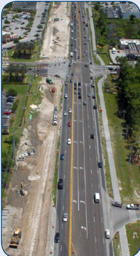
Construction of a new lane on Bruce B. Downs Boulevard between Palm Springs Road and Pebble Creek Road.
