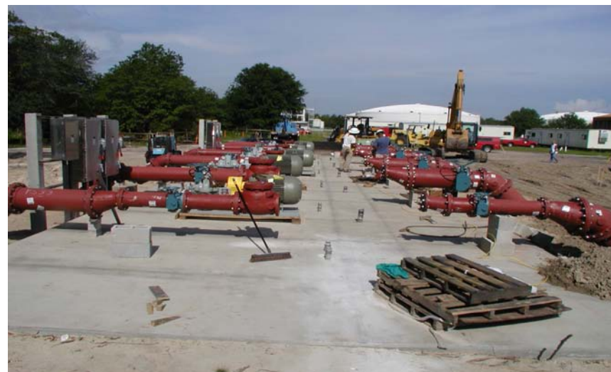
Lithia Pinecrest RW Storage and Pumping Station
