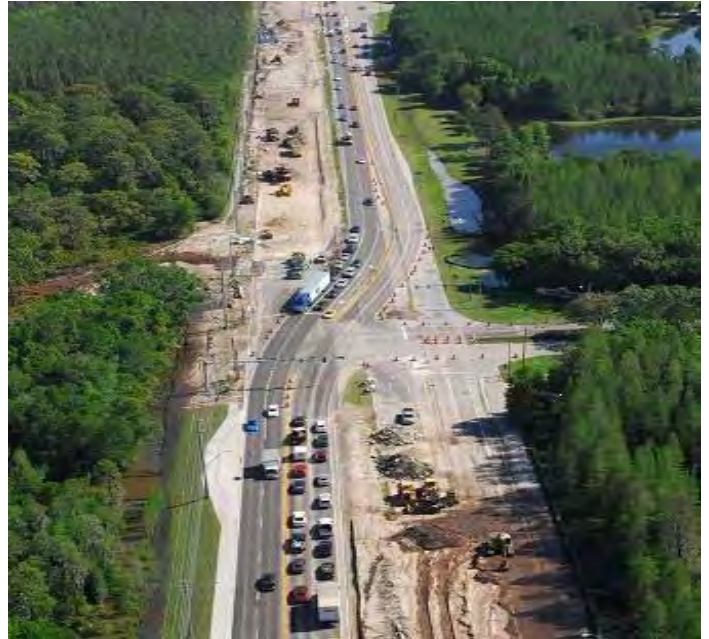
Bruce B. Downs (Palm Springs to Pebble Creek Drive South) Road Widening
